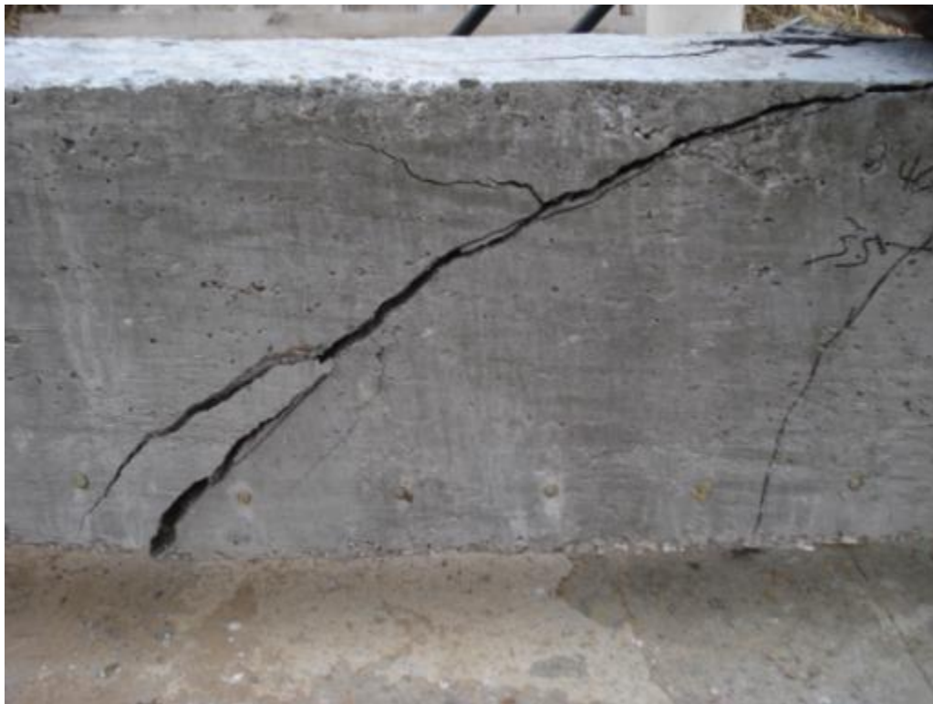
Figure 3-3. Shear/End-Slip failure of NSLS-3D (Photo by author).
